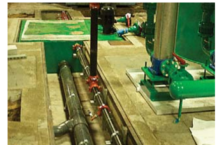
In-Ground Machine Dirty Returns to Pump-Back Sump
