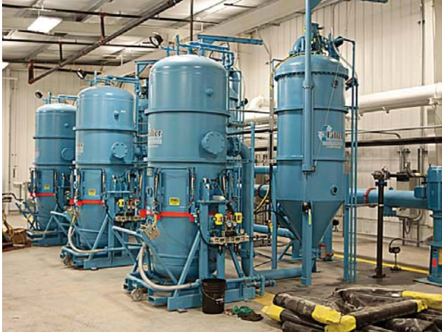
(3) 900 square foot filters and (3) sludge receivers designed with future expansion.
