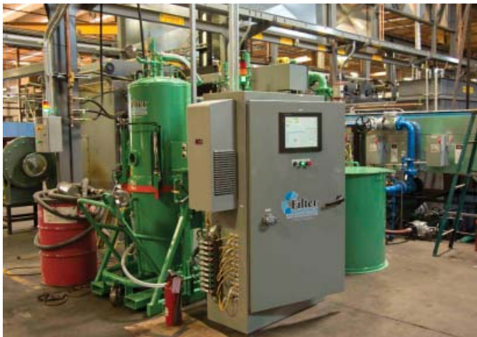
120 Square Foot Filtration System Installed and operating on an automated oil quench system.
