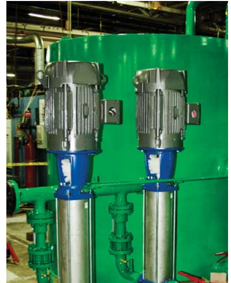
350 GPM @ 300 PSI VFD Controlled Vertical Clean Pumps.
