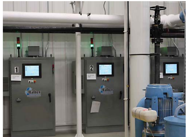
Control Panels with Color HMI Touch Screens, Data Logging, VFD Drives and Air Conditioners
