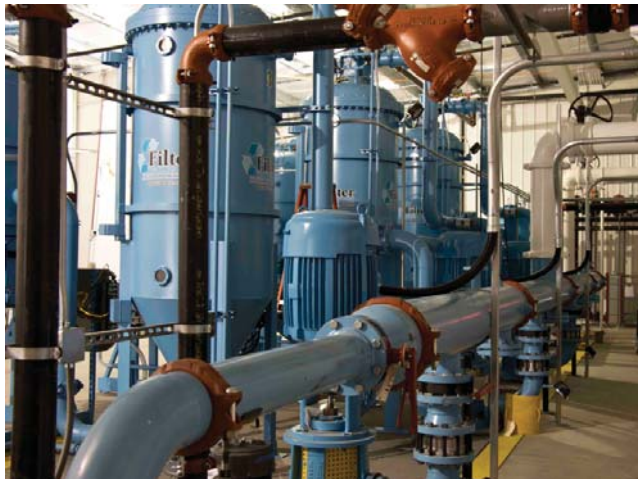
100 HP Clean Pumps with VFD Drives designed with a common manifold, check valves, and service shutoff valves for each pump.
