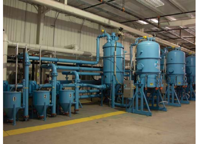
Separate filter pumps and precoat hoppers allowing for full system redundancy
