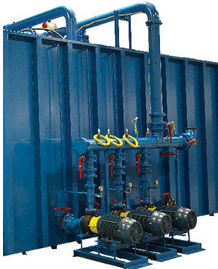
VFD Driven Multiple Clean Pumps with Standby Pump.
